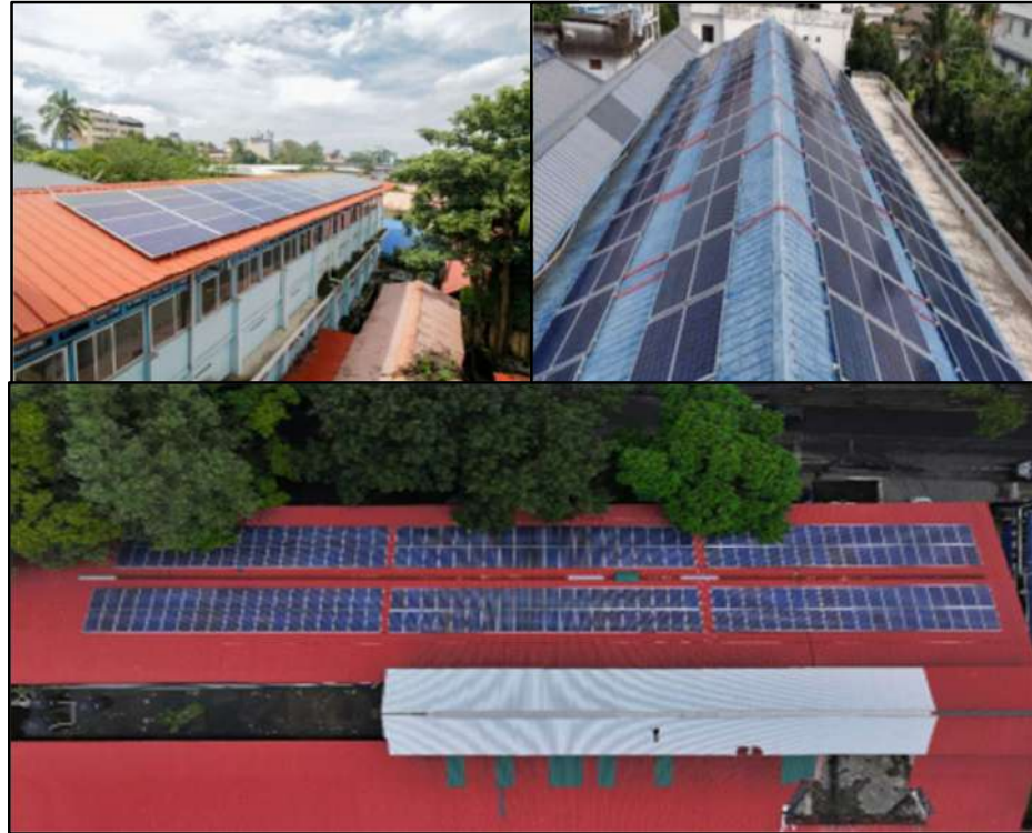
Figure 18: Roof top solar panels on Government Buildings ( Source: CSML )
