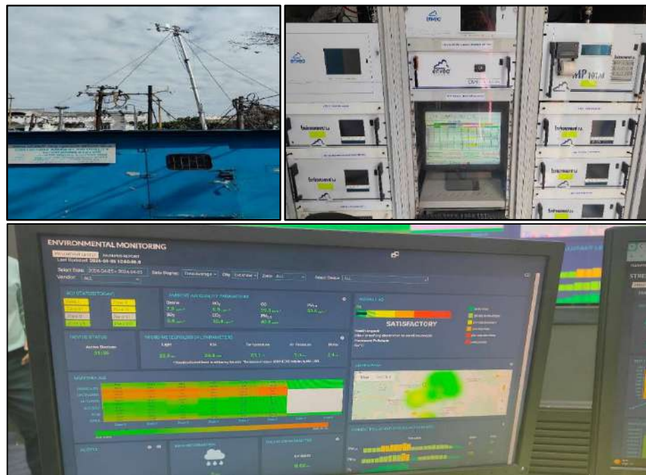
Figure 5: Environmental Sensor as seen during field visit to Lucknow (top panel) and the dashboard prepared by ICCC-Lucknow for Environmental Monitoring (bottom panel)
